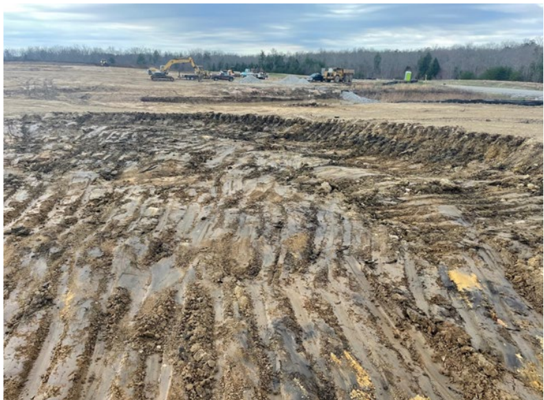
Unsuitable soil found during grading; photo taken by the construction team March 2022
